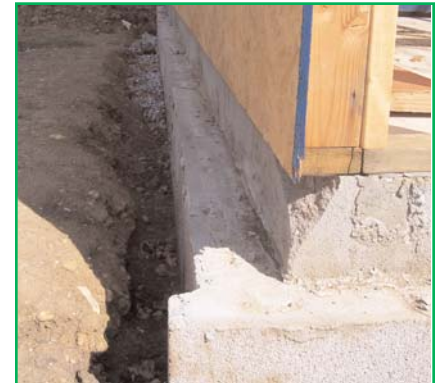
Despite having no masonry experience, students were able to lay over 700 blocks in just five hours of class time, and were able to backfill the walls the very next day!
