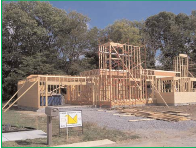
John Brown University construction management students built this home in Siloam Springs, Arkansas.
