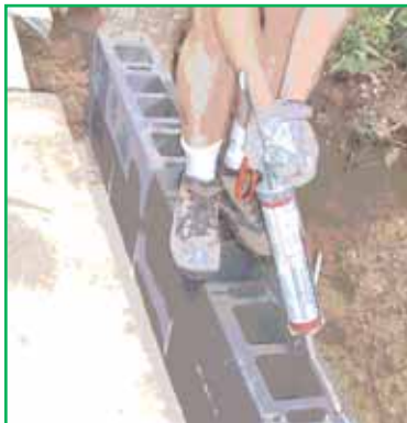
Mason Bond™ is applied to the top of the prior course, then the next course is simply stacked on top. The first course was set directly on the footing. It set quickly enough to allow Louis to stand on the course.
